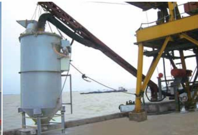
ZTG2 Ship loading system
