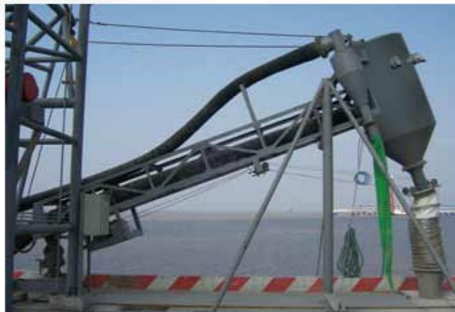
ZTG1 Ship loading system
